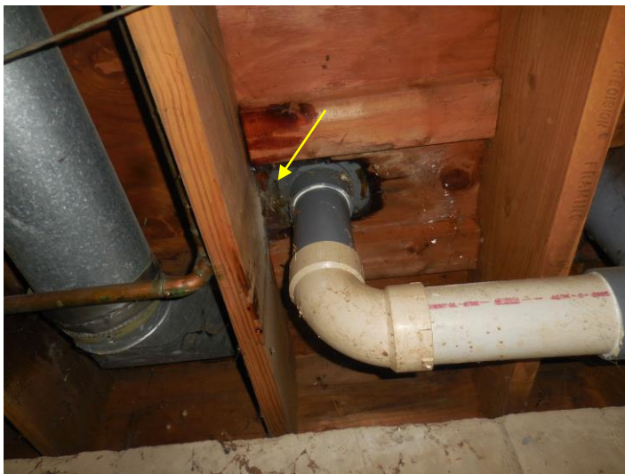
Water spilled out from underneath the flange when the master bathroom toilet was flushed
