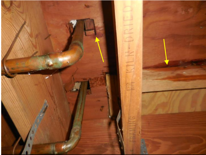
The sub-floor was wet around the water lines to the tub/shower stall in the hall bathroom.
