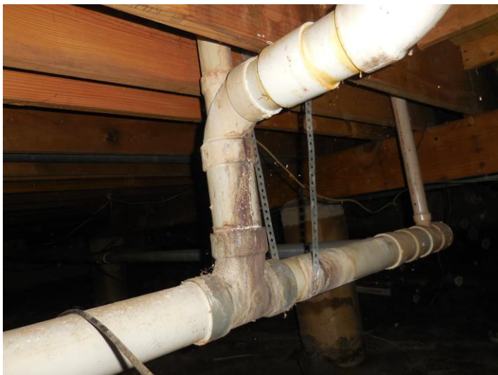
The water supply was off to the hall bathroom toilet, but it's apparent that it leaked in the past and may still be leaking
