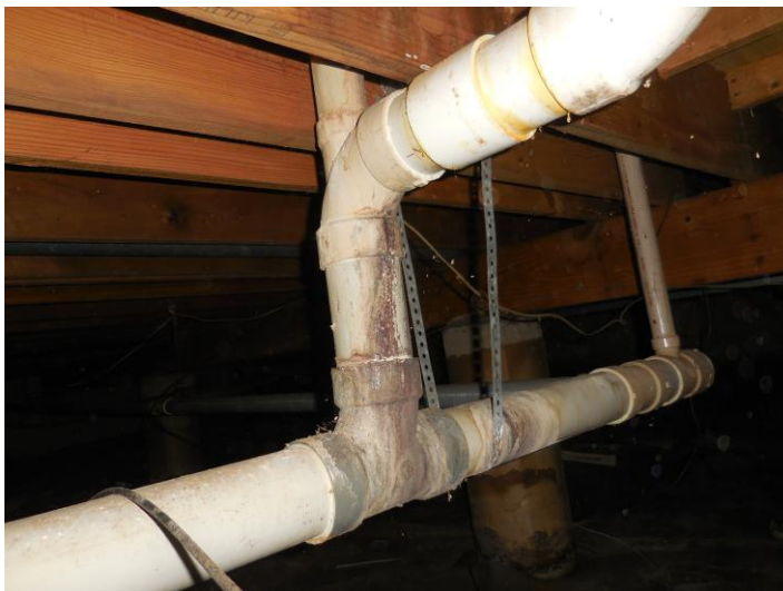
The water supply was off to the hall bathroom toilet, but it's apparent that it leaked in the past and may still be leaking
