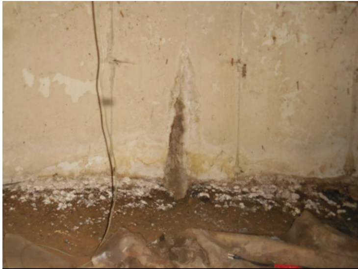
A few seeping cracks were found along the back wall of the crawlspace.
