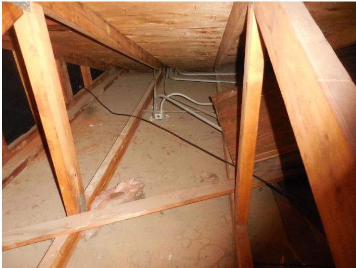
The insulation over the laundry room is missing and needs to be replaced.
