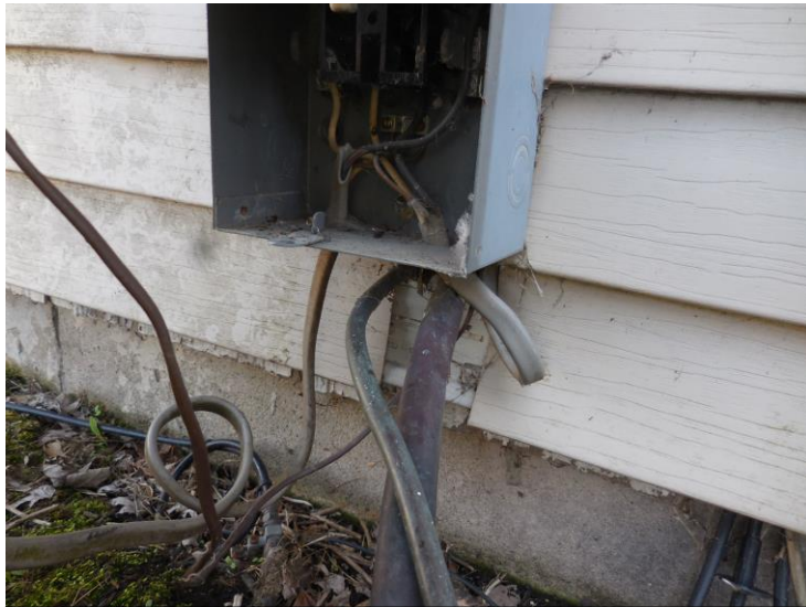
Non-professional wiring was found at the circuit for the central AC system.
