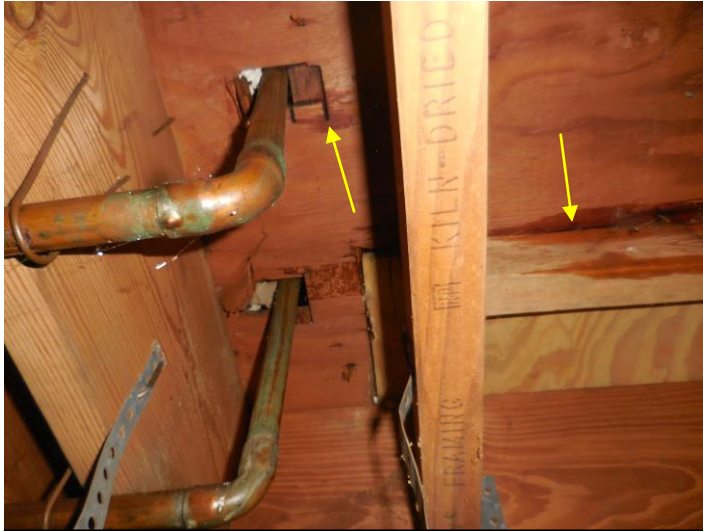
The sub-floor was wet around the water lines to the tub/shower stall in the hall bathroom.
