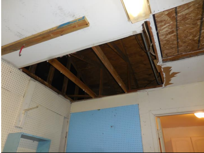
The garage ceiling needs to be repaired.
