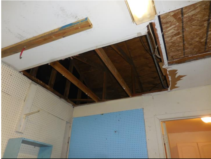
The garage ceiling needs to be repaired.
